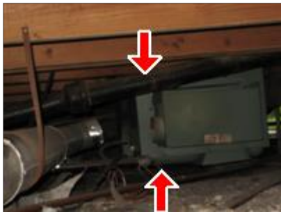
A. Picture 5 FLOOR FURNACE
