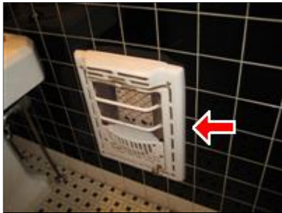
A. Picture 1 GAS WALL HEATER
