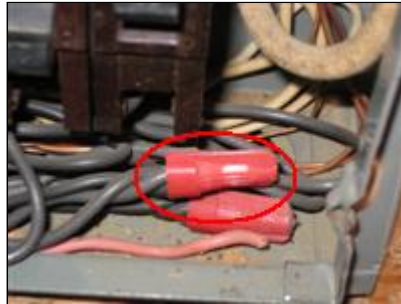
A. Picture 1 OPENING IN PANEL-BOX
