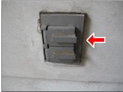
B. Picture 1 NO GFCI OUTDOORS
