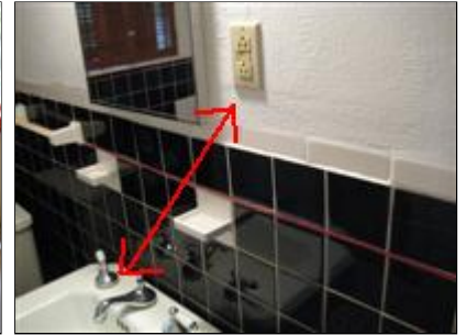
B. Picture 3 GFCI NON-FUNCTIONING
