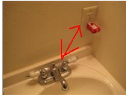
B. Picture 4 NO GFCI IN BATHROOMS
