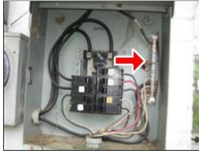
A. Picture 9 SUB-PANEL OUTSIDE
