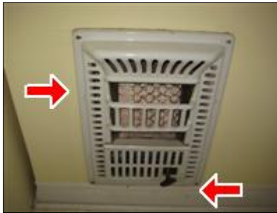
A. Picture 2 DISALLOWED BY STANDARDS
