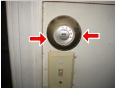
A. Picture 4 NON-FUNCTIONING
