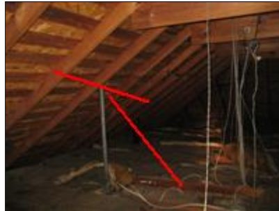
D. Picture 4 LACK OF RAFTER SUPPORTS
