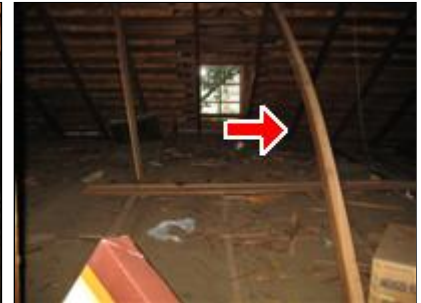
D. Picture 5 WEAK / UNSTABLE SUPPORTS
