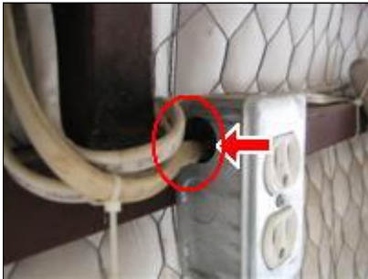
B. Picture 9 No wire-stop at metal boxes
