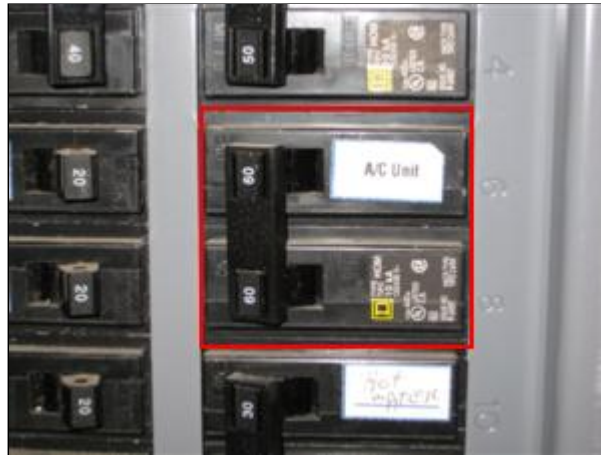
B. Picture 17 Breaker to Main Condensing-unit
