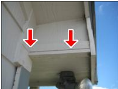
E. Picture 1 OPENINGS IN SOFFIT
