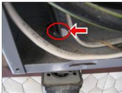
B. Picture 12 Panel Box at detached garage
