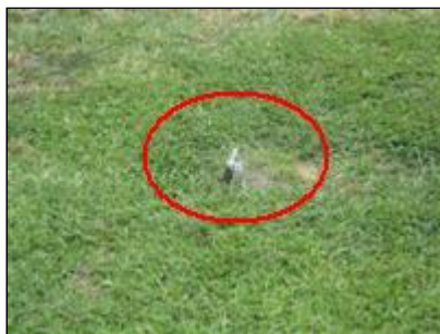
A. Picture 4 Zone# 9 damaged heads
