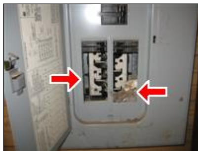
A. Picture 2 SUB-PANEL IN STABLES
