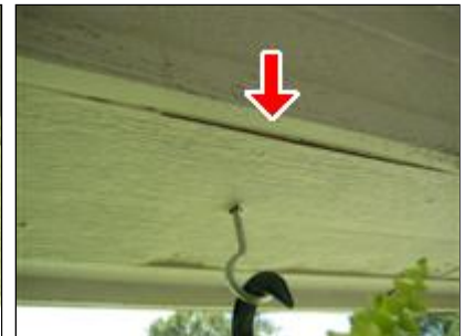
E. Picture 3 SEAM OPENINGS
