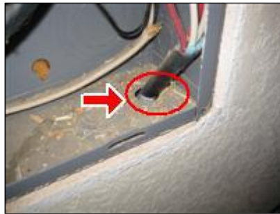
B. Picture 7 Panel Box at House
