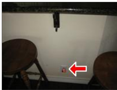
B. Picture 14 NO GFCI UNDER BAR
