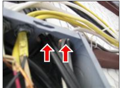
B. Picture 11 Panel Box at detached garage
