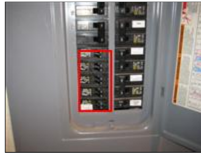
B. Picture 22 Missing AFCI Breakers
