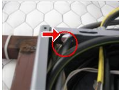
B. Picture 10 Panel Box at detached garage
