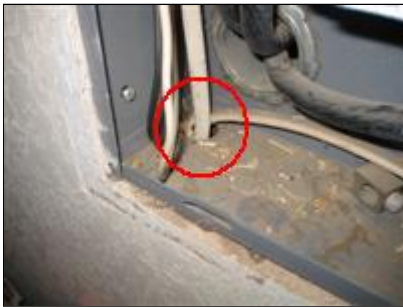
B. Picture 6 Panel Box at House
