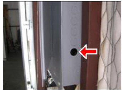
B. Picture 8 Panel Box at detached garage
