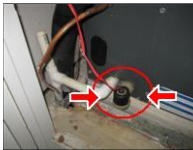
B. Picture 2 Water Overflow Sensor
